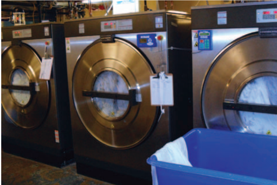
These 130-pound capacity Continental L-Series allowed the Westin Riverwalk Hotel to receive a rebate from the San Antonio Water System and dramatically cut water costs.
