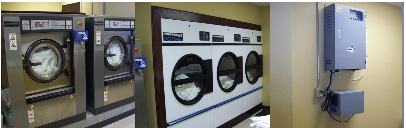
Every system in the Hilton Garden Inn Gatlinburg was examined in order to heighten hotel sustainability, even the in-house laundry, which comes complete with an ozone system, soft-mount, high-speed washer-extractors and high-efficiency dryers. In five years, the laundry alone is expected to save the hotel $60,196.
